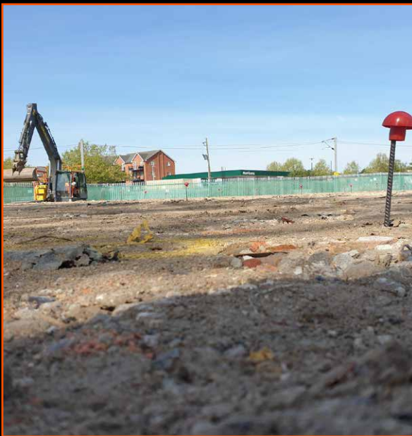
Primary Site Control Establishment, Setting Out Services Including grid lines and piling locations, Vibration Monitoring, Structural Monitoring, Topographic Survey
